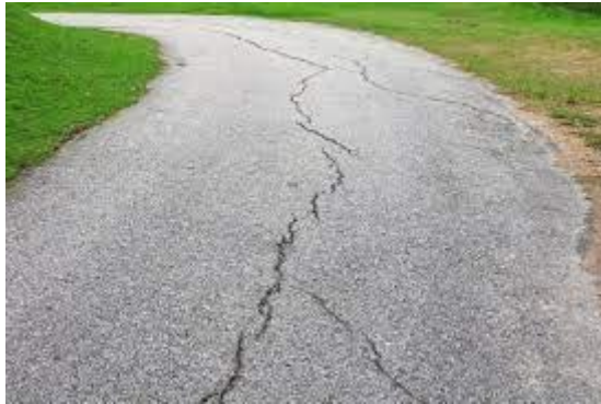
Figure 4: The above diagram shows the distortion, which is defined as the change of real road to any other shape due to heavy, loads [ilpaving].
